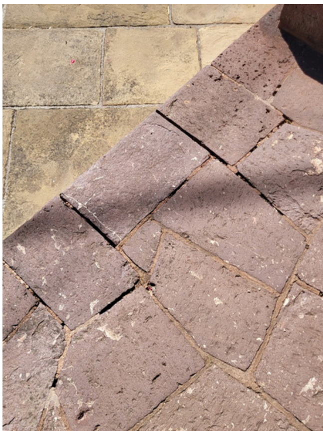
Image 3: Small sections of internal slabs need repointing
