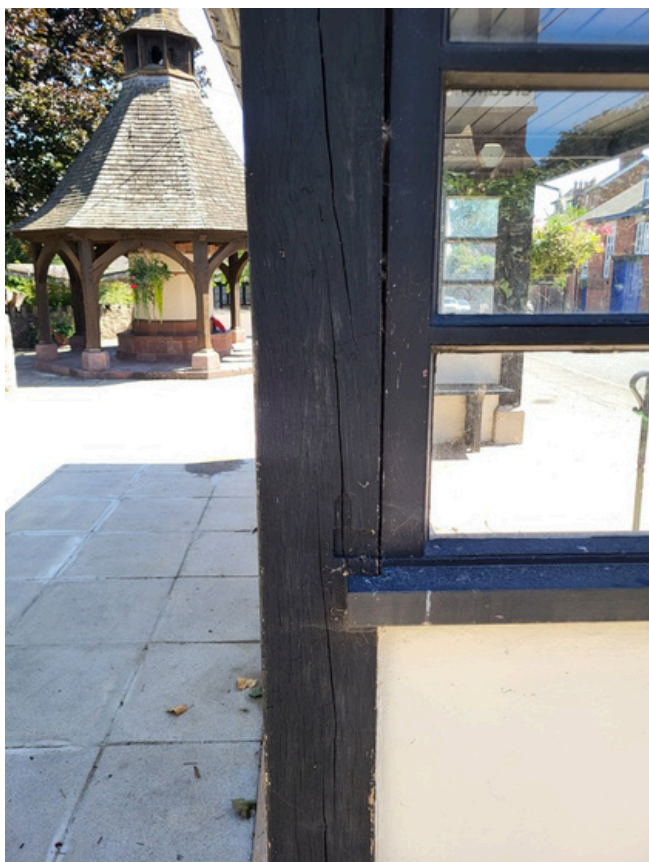
Image 11: No change in cracks to uprights
