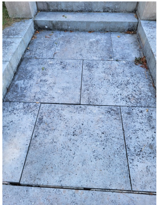
Image 4: Loose pointing on steps
