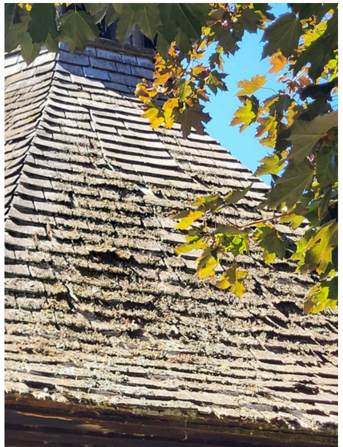
Image 13: Rear elevation - large amounts of moss and more significant warping
