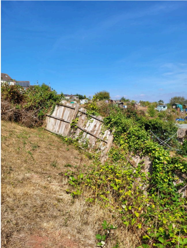
Image 5: Fence requires attention - housing association to repair
