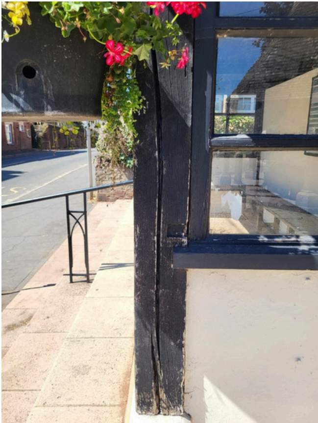
Image 9: No change in cracks to uprights
