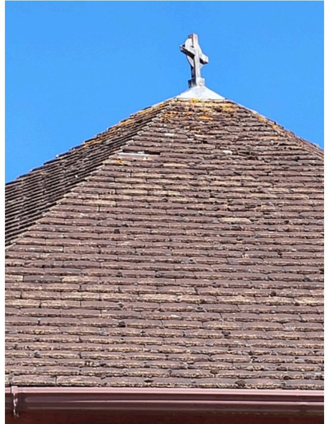
Image 2: One missing tile at the rear
