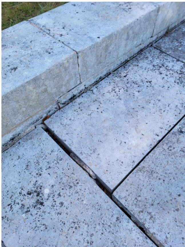
Image 3: Loose pointing on steps
