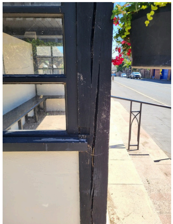
Image 12: No change in cracks to uprights
