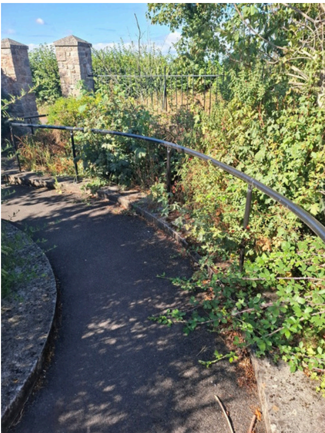
Image 7: Shrubs beginning to encroach onto path, due to be cut back on next visit
