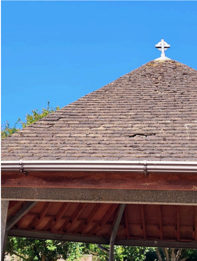
Image 1: Two missing roof tiles at the front
