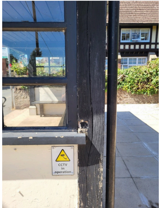
Image 10: No change in cracks to uprights
