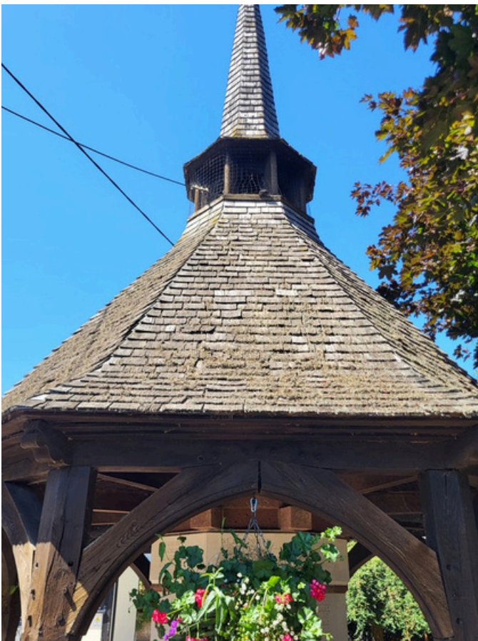
Image 12: East elevation - roof shingles starting to warp
