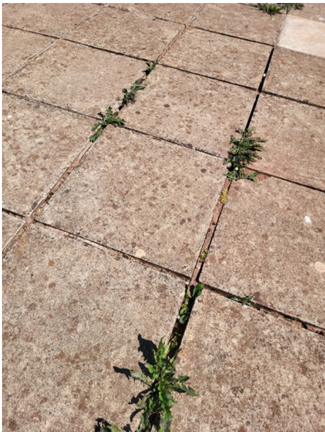
Image 3: Loose pointing and weeds
