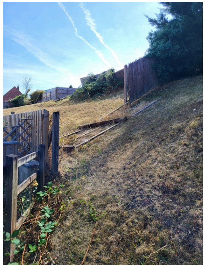
Image 4: Fence requires attention - housing association to repair
