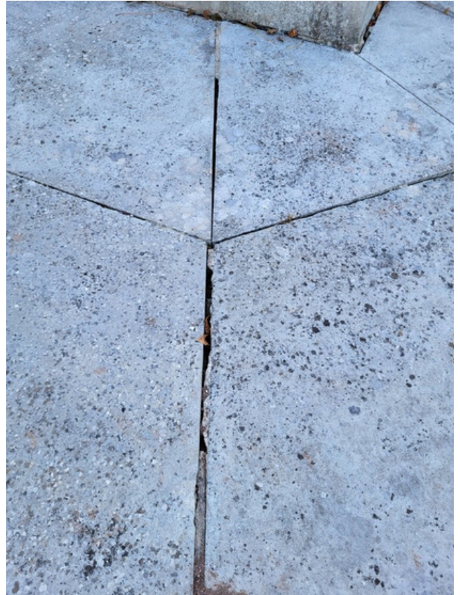
Image 2: Loose pointing around statue
