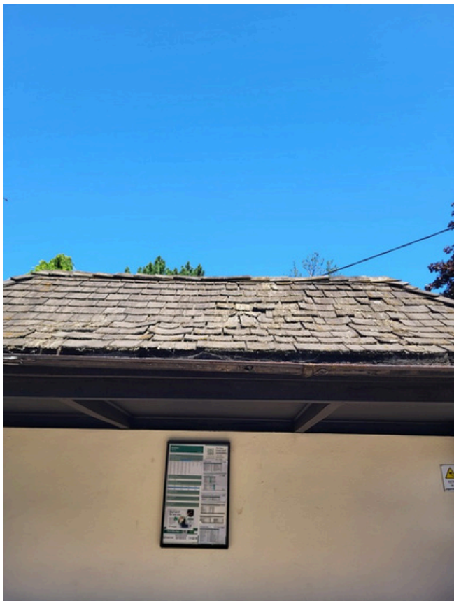
Image 7: Warped roof tiles
